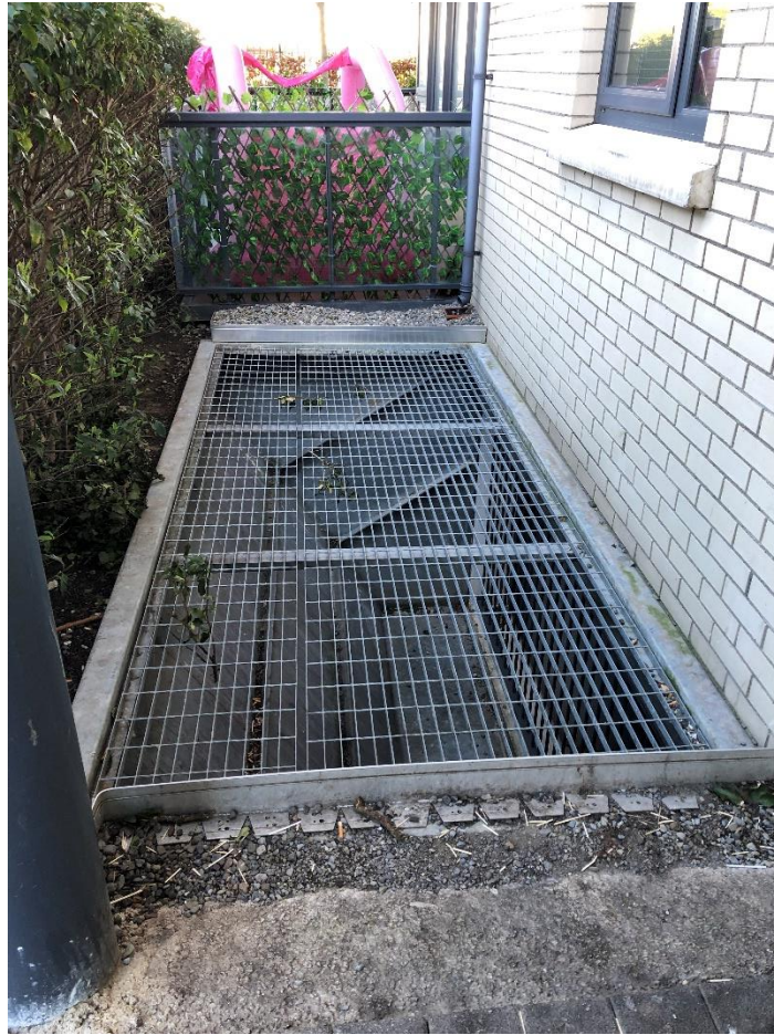
Plantroom Ventilation opening
