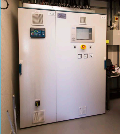
Bausch + Lomb CHP Controller
