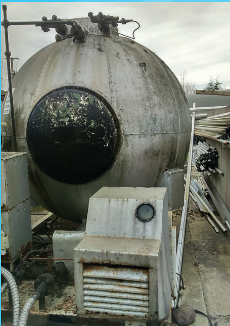
The old CO 2 tank that is no longer needed
