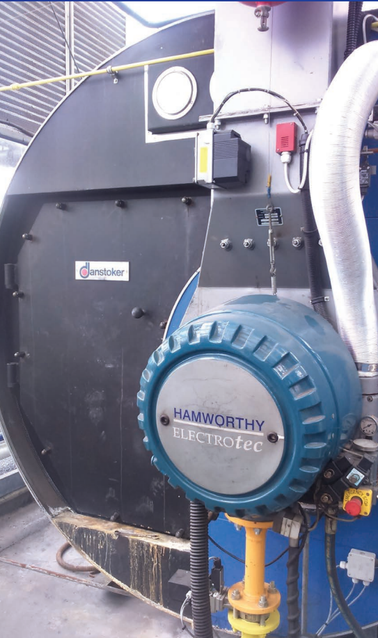
Natural gas boiler and burner
