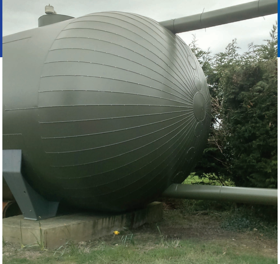
Hot water storage tank
