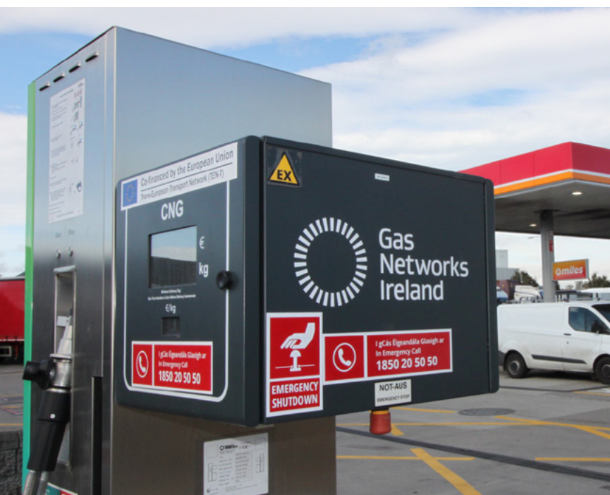
Figure 8-1: Dublin Port CNG Station
