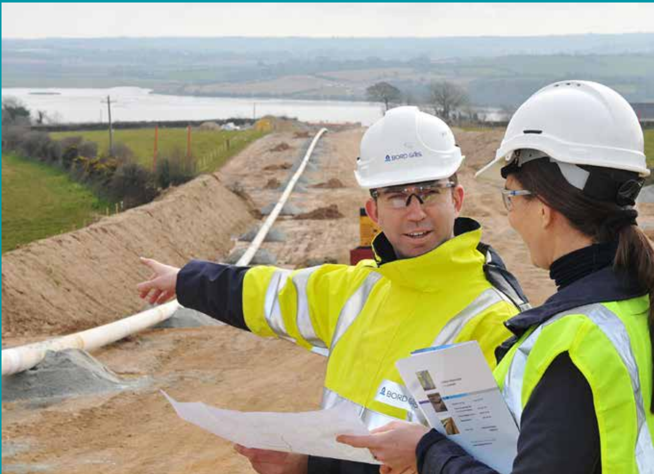
Denis Barry, Senior Asset Programme Manager, Bord Gáis Networks and Linda O'Brien, Community Liaison Officer, Bord Gáis Networks on site at the river crossing works on the Gas to Great Island Project.
