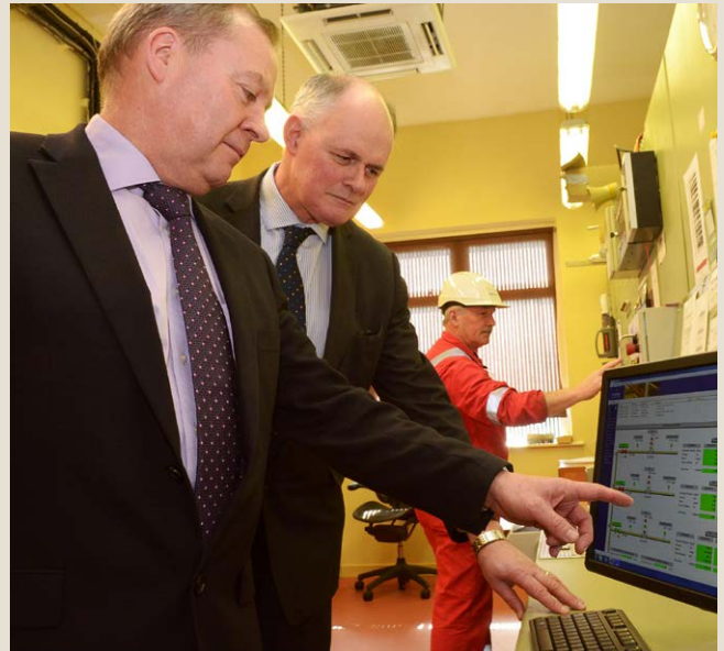
CEO Kinsale Energy, Fergal Murphy and Gaslink GM, Aidan O'Sullivan at the Inch Control Room
