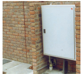
Six meter cabinet
