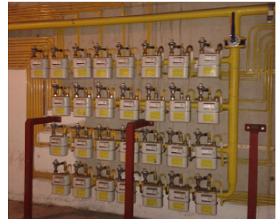
On-site meter manifold
