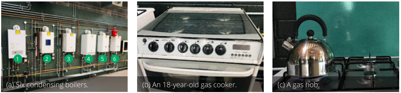
Figure 3. Appliances; (a) six condensing boilers, (b) an 18-year-old gas cooker, (c) a gas hob.
